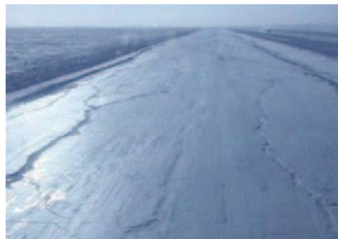
Normal longitudinal cracking caused by buoyancy of the thickened ice over the 20-metre-wide travel lane
