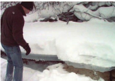
Hinge crack that became a break along a lake shoreline when the water level dropped
